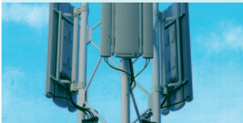
in transmitter stations of cellular phone networks
